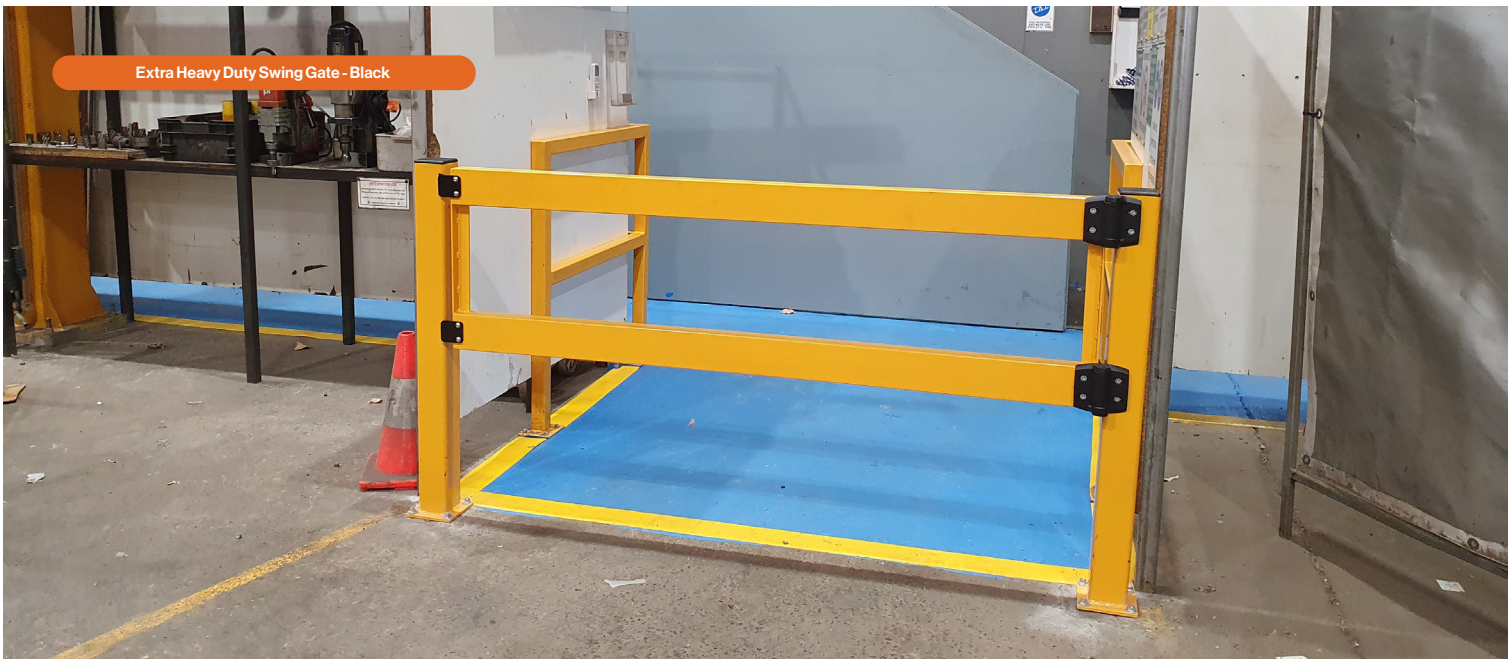
Recessed Rail Pedestrian Gates - Alarmed
